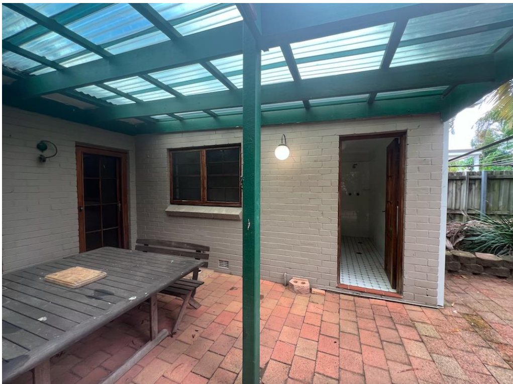
Figure 34 – Rear patio area, with entrance to rear laundry, windows and doors to be replaced (Source: Three + One Heritage, 2024)
