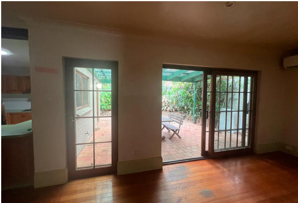
Figure 32 – Doors onto rear patio, to be replaced (Source: Three + One Heritage, 2024)
