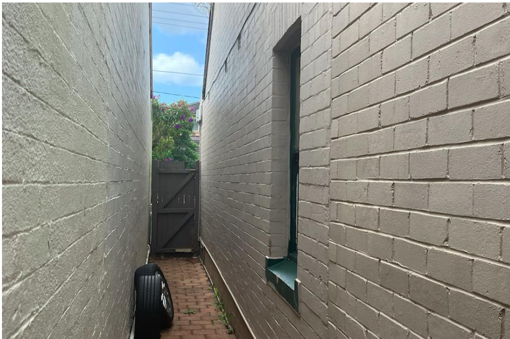
Figure 38 – Northern side passage, view looking east towards Gordon Street, location of previous rear extension visible in changes to brickwork (Source: Three + One Heritage, 2024)
