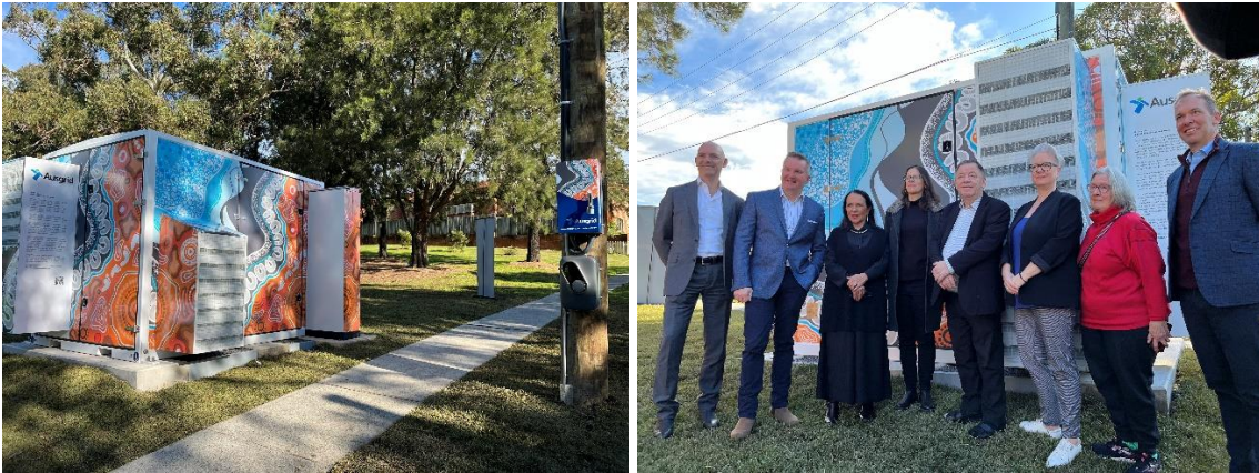
Figure 2: Community Battery and pole-mounted EV charging station at Gilchrist Park, Bexley North
