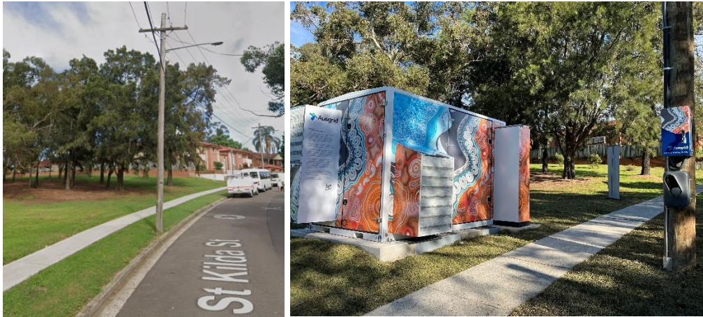
Figure 1: Community Battery and pole-mounted EV charging station at St Kilda St Bexley North
